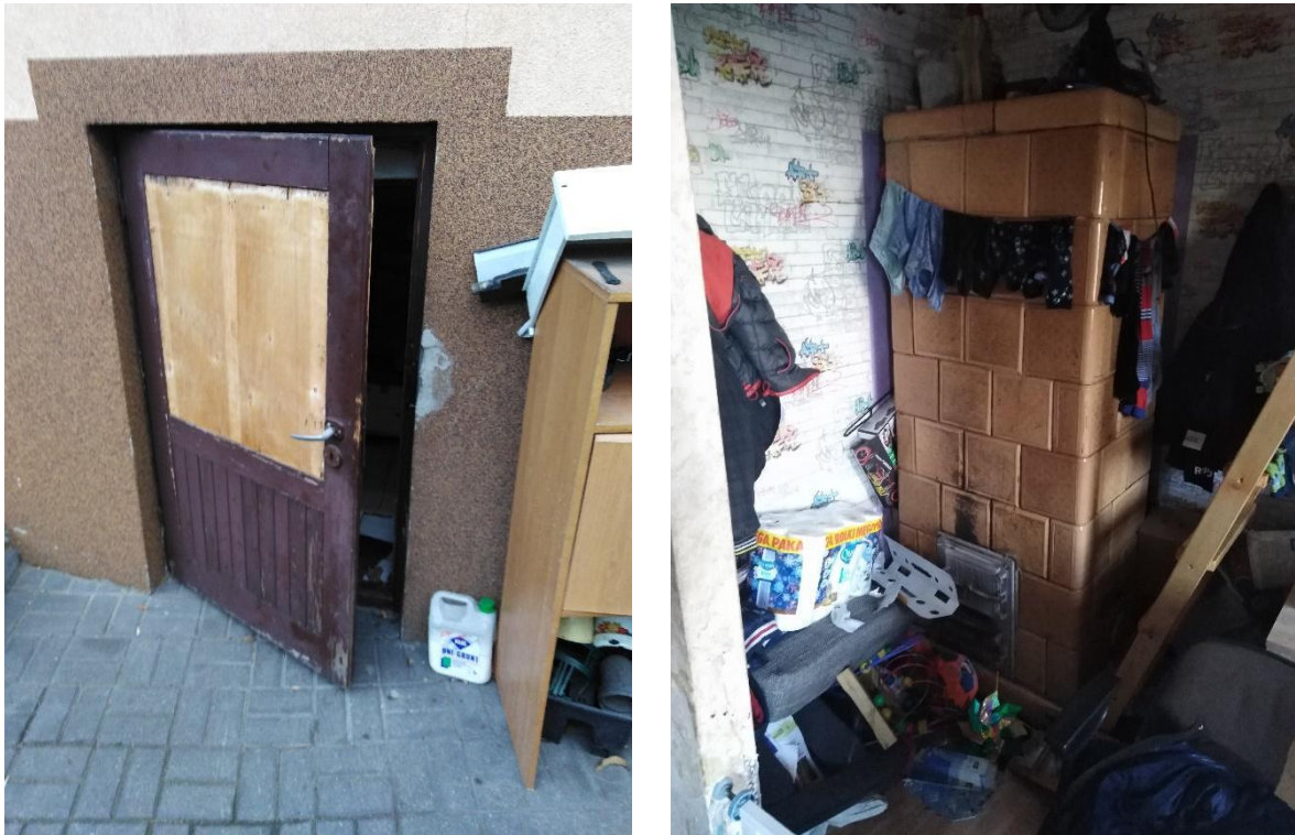
Photo 2: Left: Temporary covering of defects in the door to the boiler room using plywood. Right: A working coal tiled stove next to a children's bunk bed.
